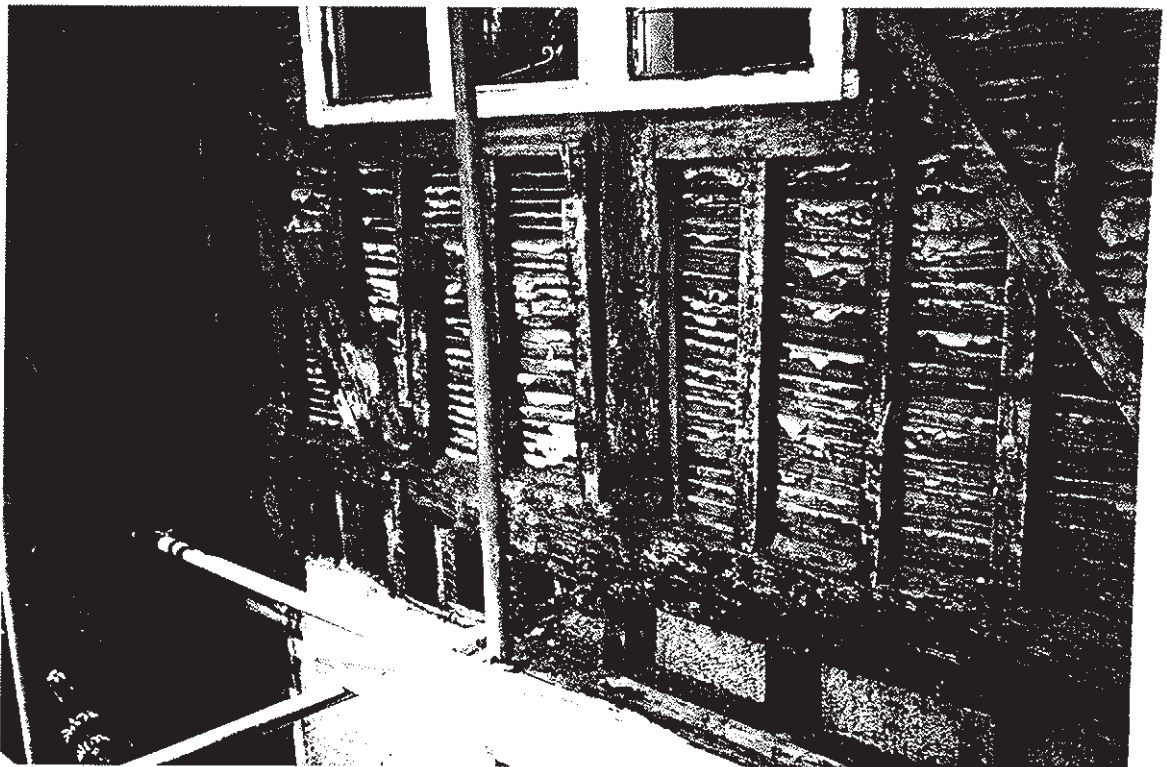
Plate 10: East wall, south rear wing: note lack of mortices in principal joist.
